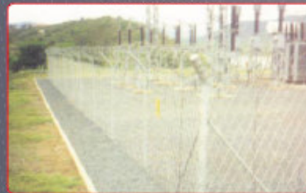
ELECTRICAL SUB STATION
